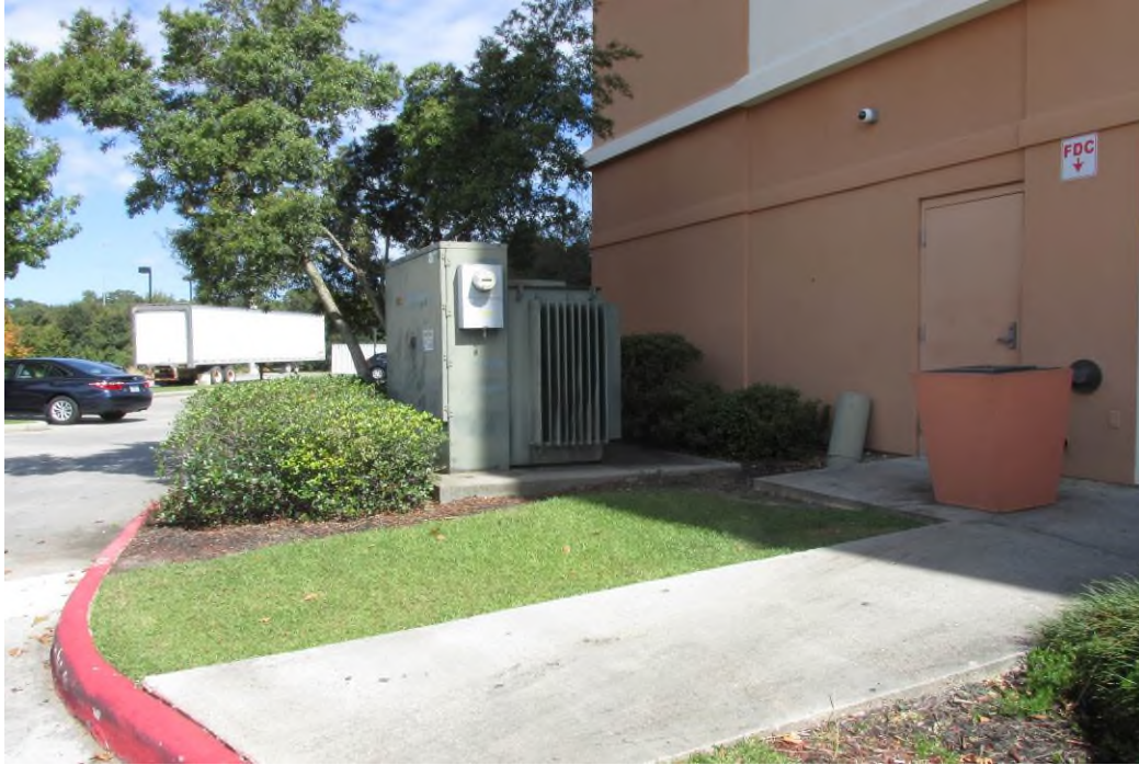
Electric vault extends 11 feet from Hyatt side door
